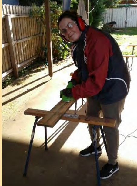
Casey sanding the fence paling ready for a fresh coat of paint.
